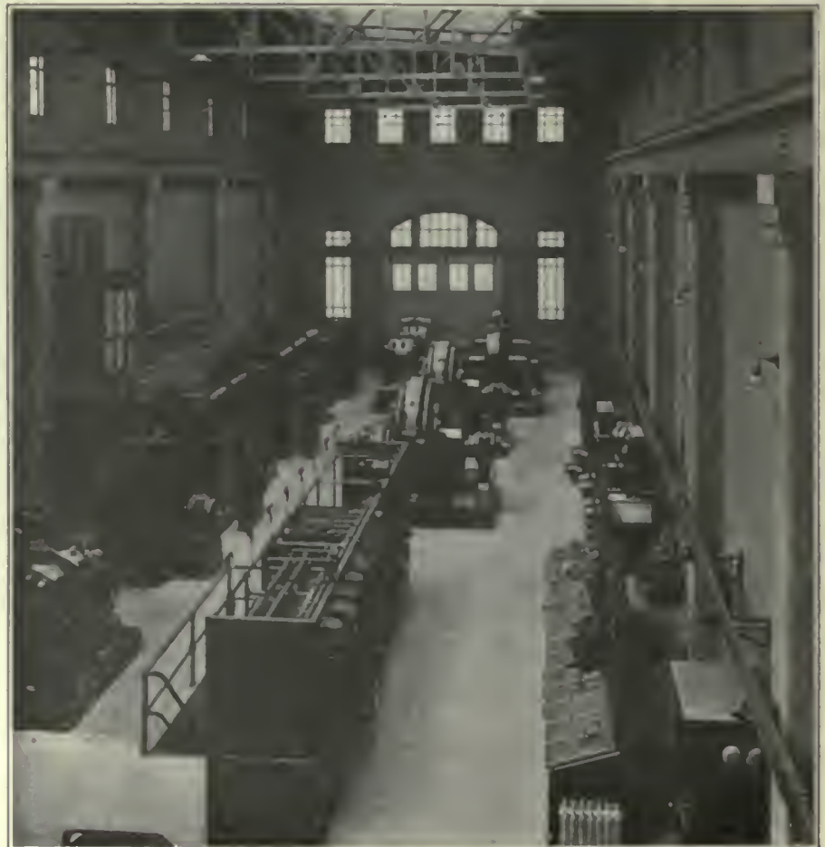
FIG. 496. SUBSTATIONS. Interior View of Substation of the New York Central & Hudson River Railroad.
